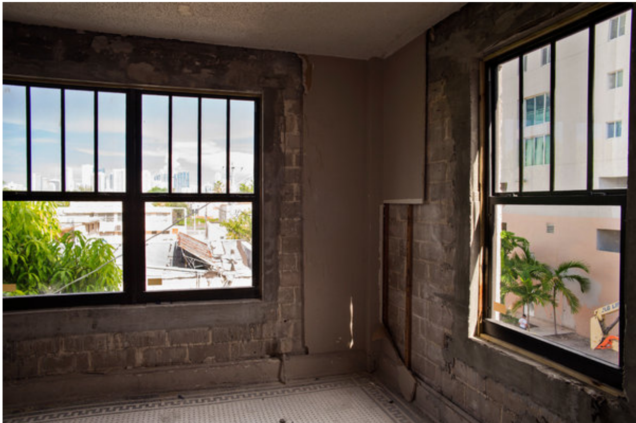
A room in the Tower Hotel in Little Havana, which is under renovation. ÁNGEL FRANCO / THE NEW YORK TIMES
